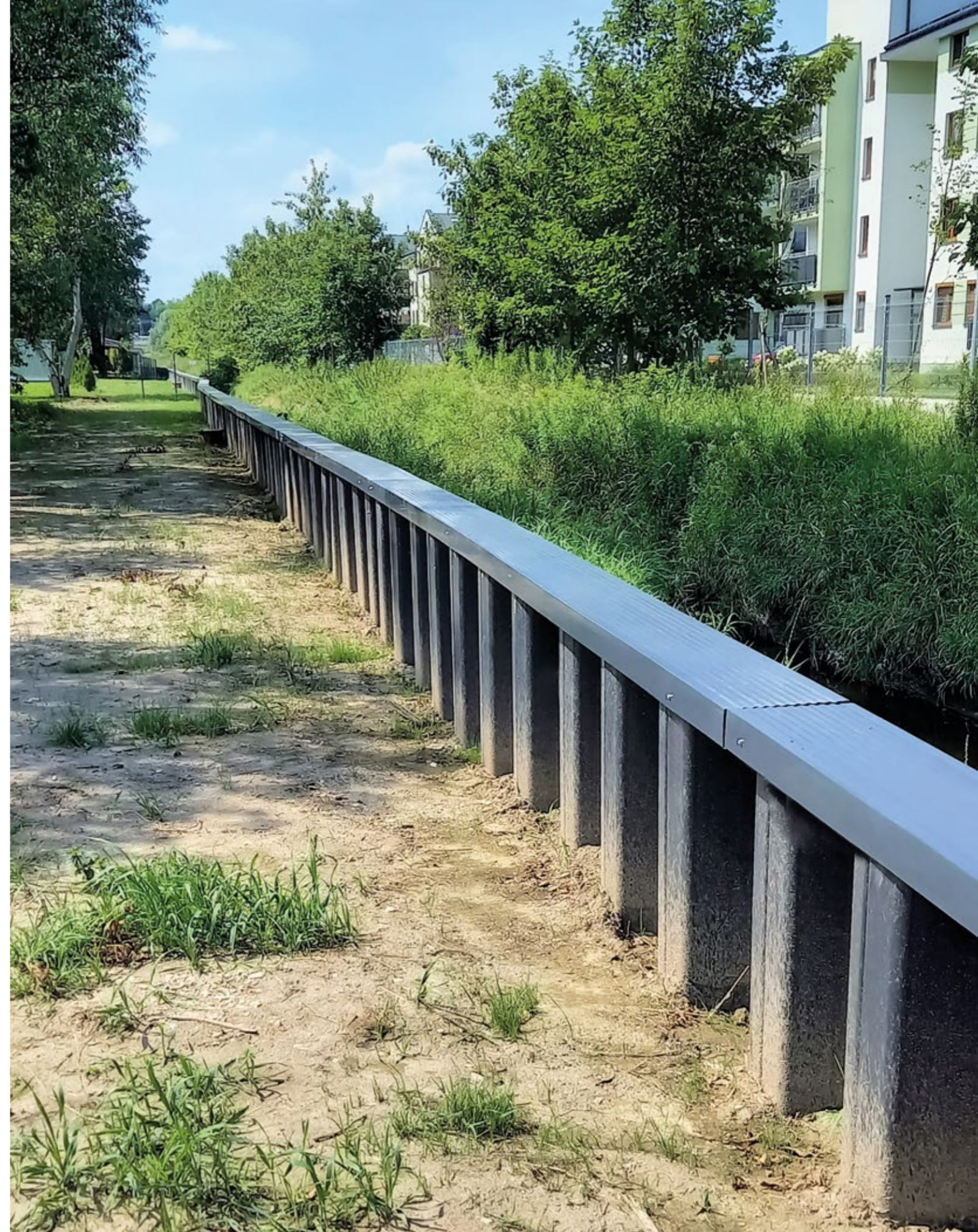
CRACOW, POLAND: VINYL SHEET PILES USED AS AN ELEMENT OF FLOOD PROTECTION INFRASTRUCTURE IN A DENSELY URBANIZED AREA.
