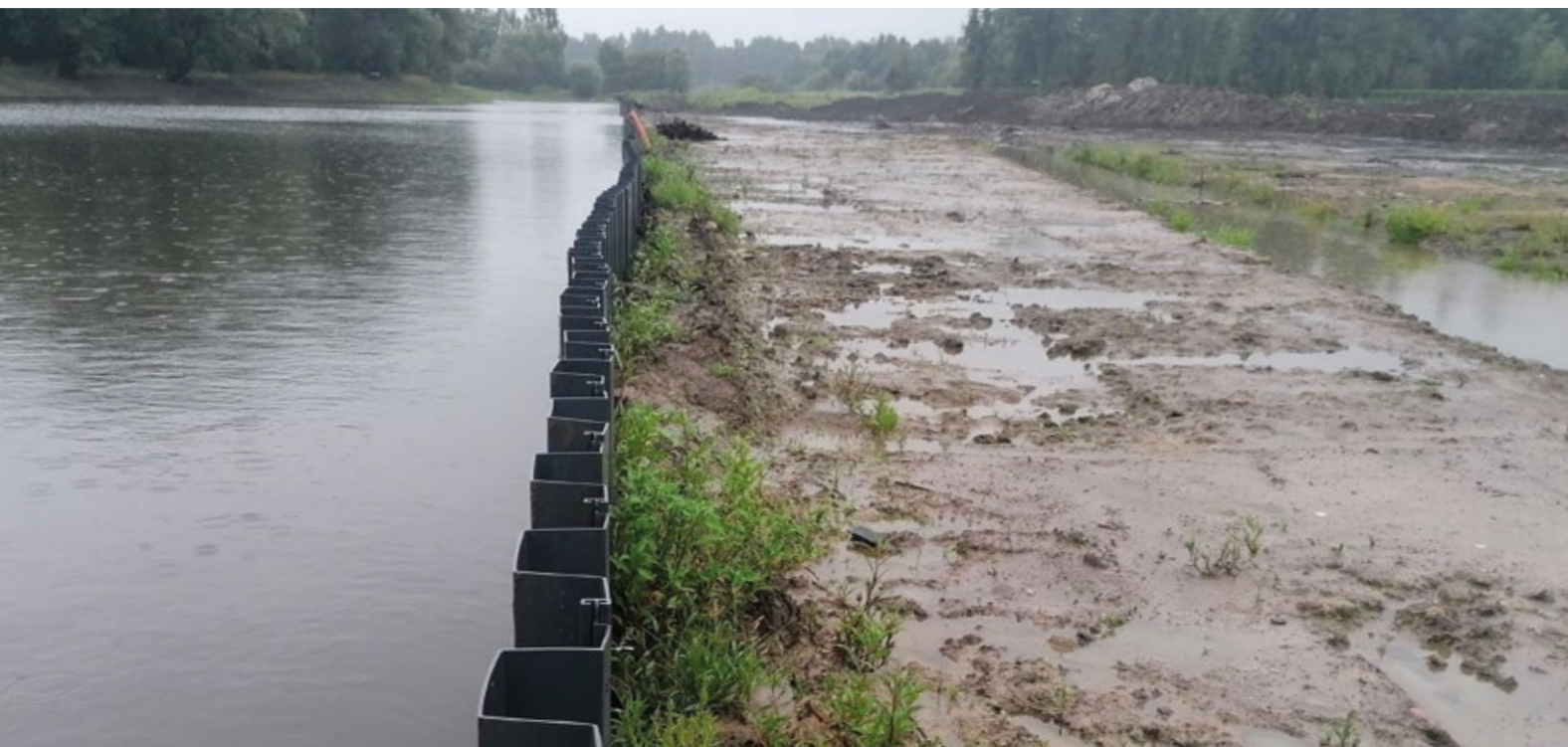
KOMORÓW, POLAND: VINYL SHEET PILES WITH GASKETS USED TO TEMPORARY REDIRECT THE RIVER BED.
