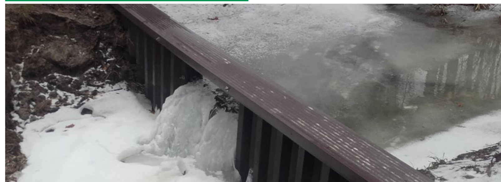
THE PODANIN FOREST DISTRICT, POLAND: VINYL SMALL RETENTION SLUICES ARE DURABLE AND RESISTANT TO ATMOSPHERIC CONDITIONS.
