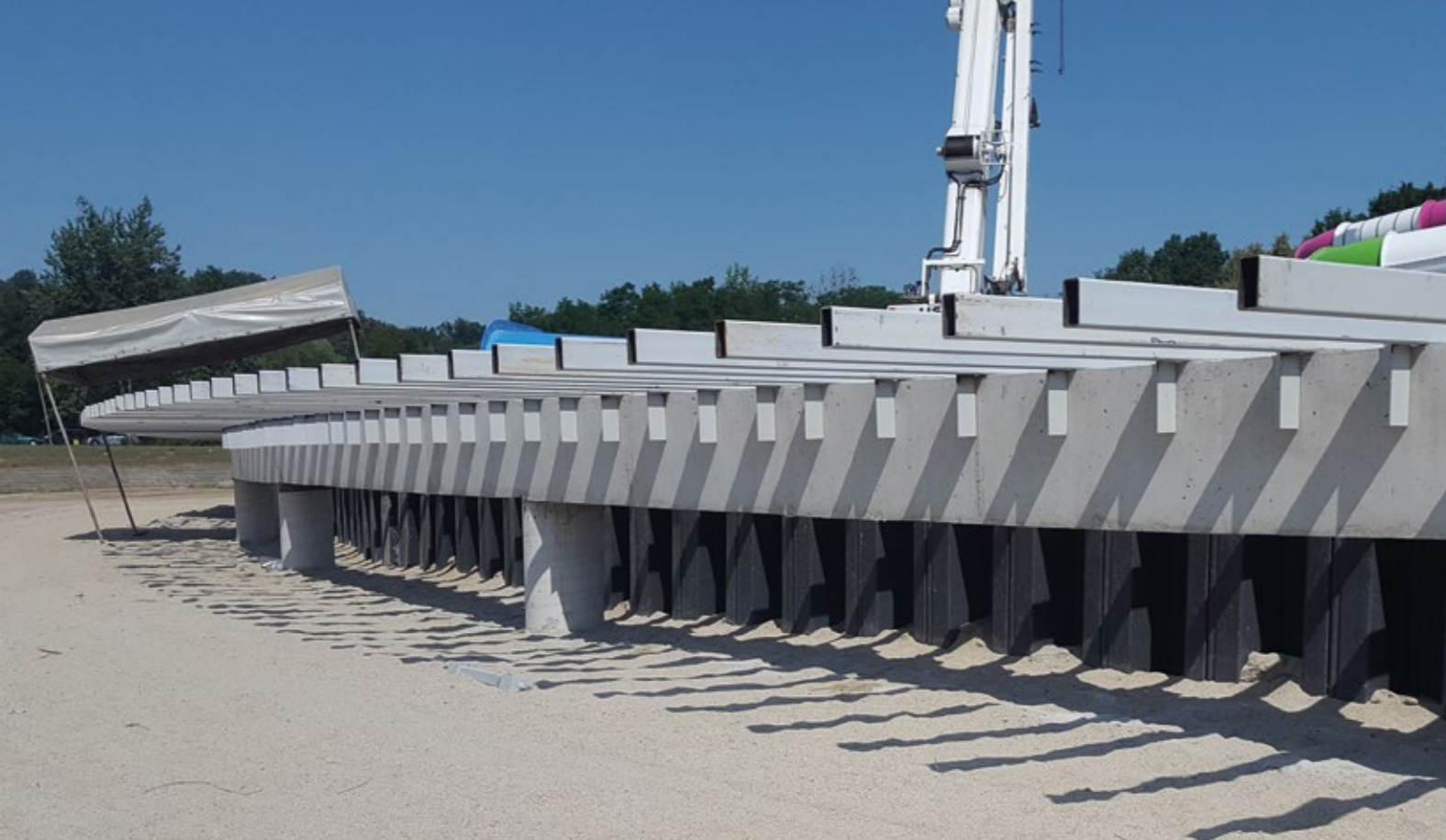
NYSA, POLAND: VINYL SHEET PILING USED TO CONSTRUCT A MUNICIPAL WATER PARK.
