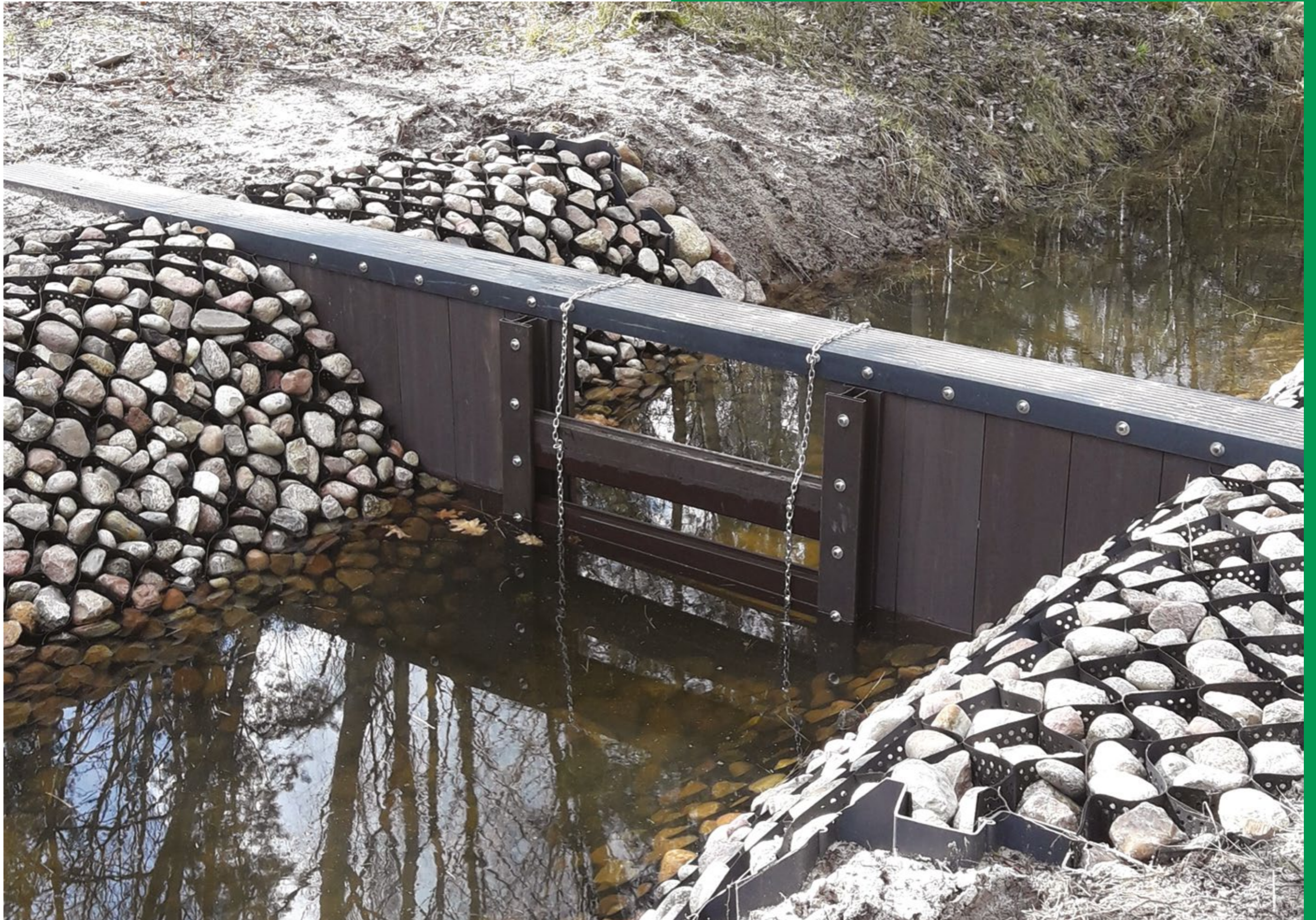
GRABÓW, POLAND: AN ELEMENT OF A COMPREHENSIVE WATER RETENTION SYSTEM IN THE PILICA RIVER BASIN.
