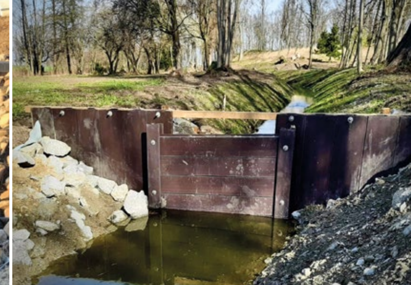
THE JAROCIN AREA, POLAND: SMALL RETENTION SLUICES INSTALLED IN A DEVELOPMENT PROJECT OF A MUNICIPAL PARK.
