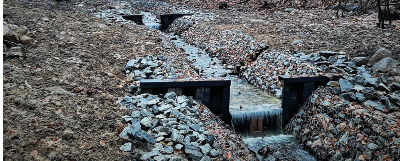
SZCZECIN, POLAND: WATER BARRAGES MADE OF VINYL SHEET PILES FINISHED WITH A CAP.
