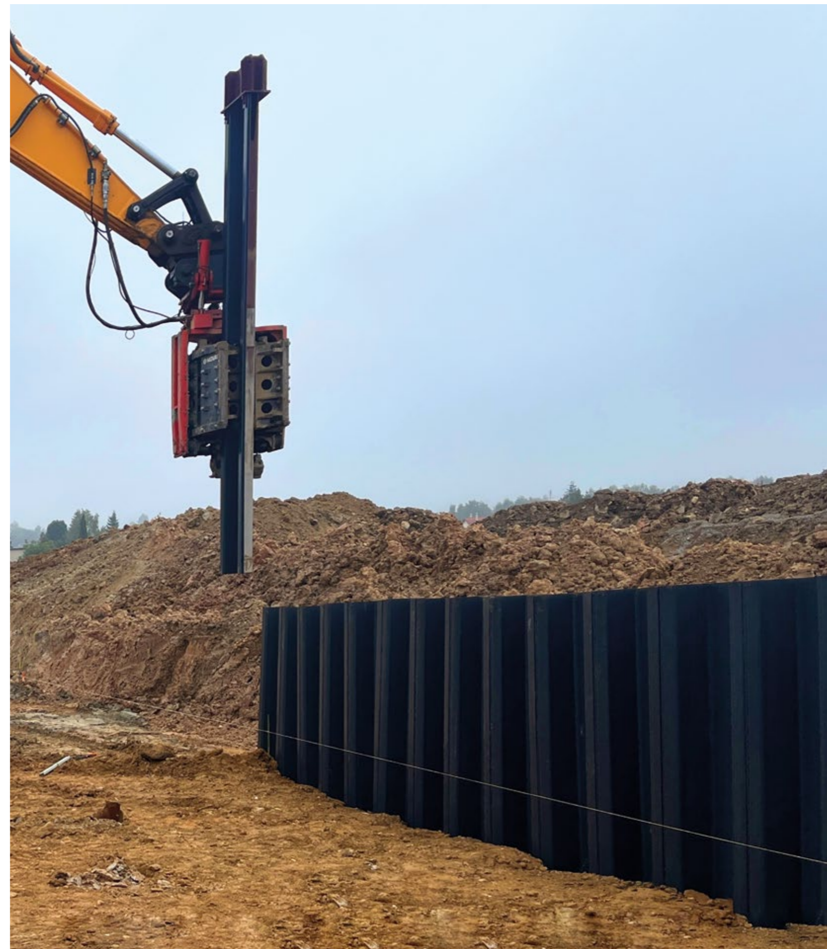
BUDEJOVICE, CZECH REPUBLIC: INSTALLATION OF VINYL SHEET PILES IN DIFFICULT SOIL CONDITIONS.
