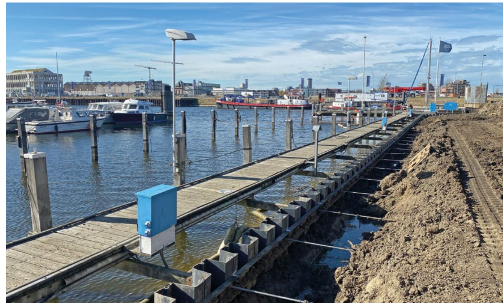
VLISSINGEN, THE NETHERLANDS: VINYL SHEET PILING WALL REINFORCED WITH EARTH ANCHORS IN A HARBOUR DEVELOPMENT PROJECT.
